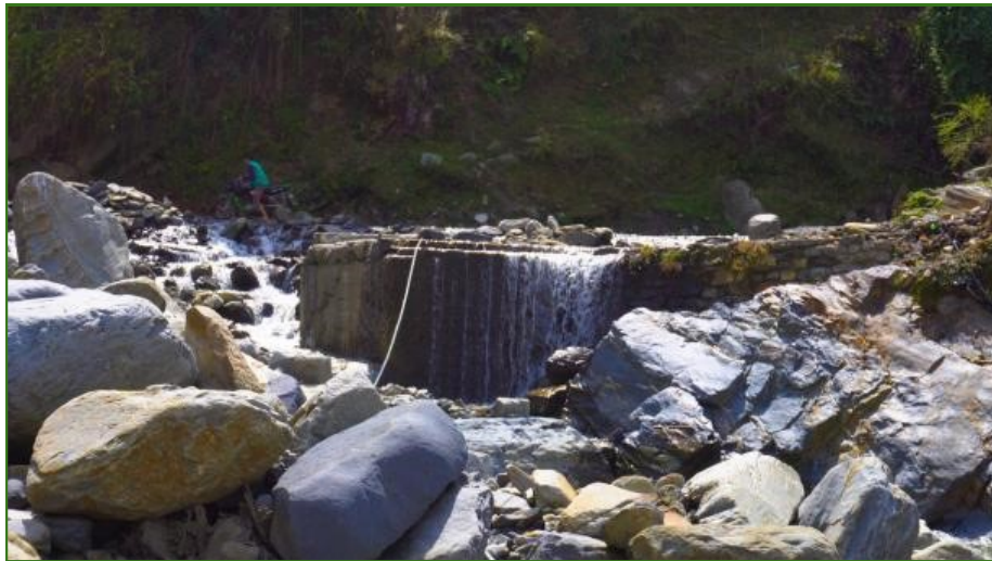
Figure 1: Remnants of a bridge destroyed in a flash flood in Bagi village (Photo by Brant Reymann).
